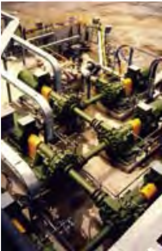
Pressure booster station (Warman)
